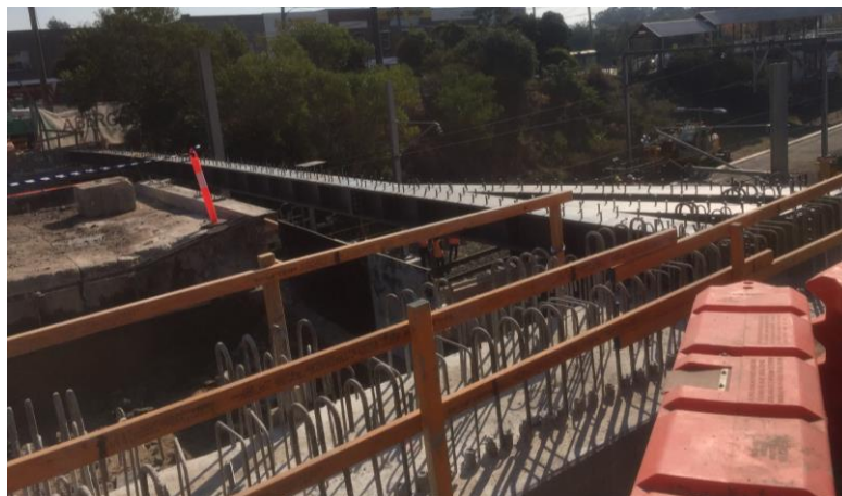
Figure 12. Installation of outer steel girders to allow for removal of central masonry pier at second track possession
