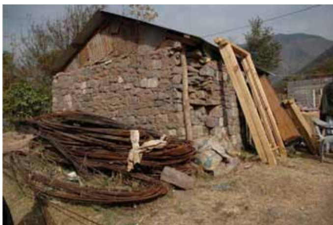
a) A stone masonry building with light timber frame, damaged by earthquake.
