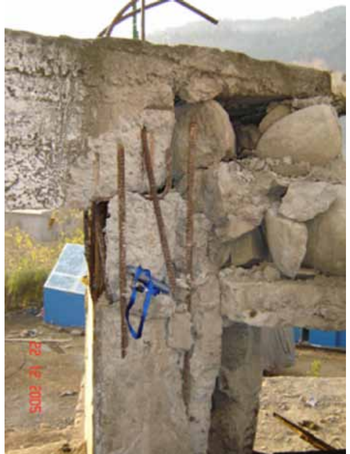
d) No stirrups in column.
