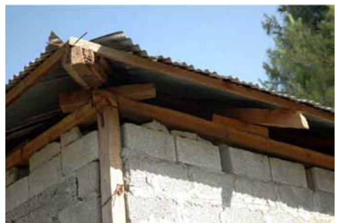
b) A block masonry building with light timber frame constructed after earthquake (note change in walls after earthquake).
