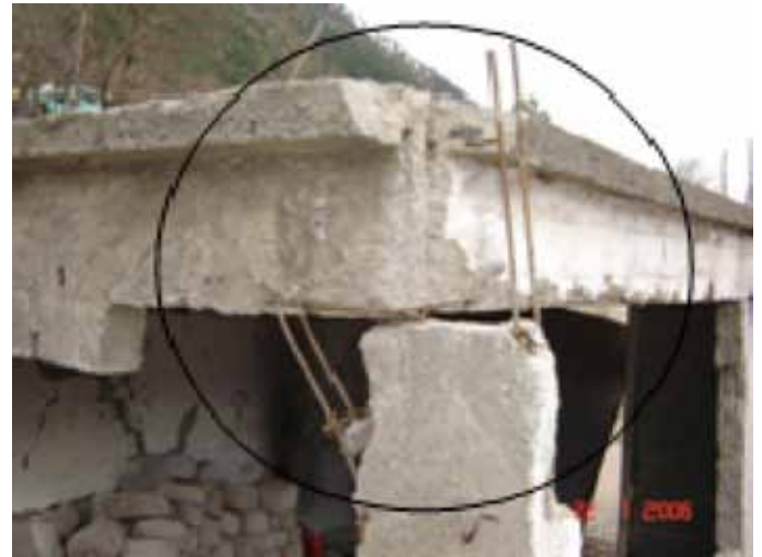
c) Cold-joint problem.
